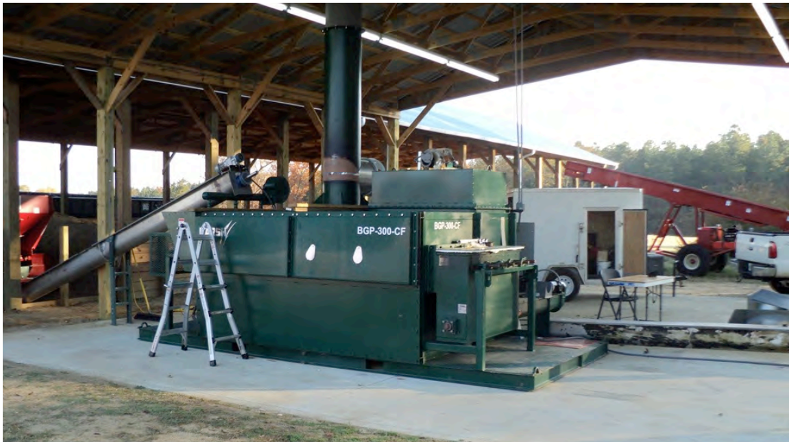
Gasifier that consumes poultry litter and generates electricity at the Marc Marsh Farm in Cheraw, SC; Source: FPPC
